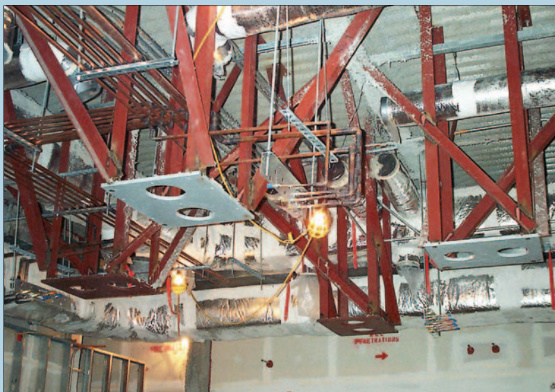
▲ FROM BEAMS TO BOOMS Make sure your facility's superstructure can support the weight of ceiling-service booms.
